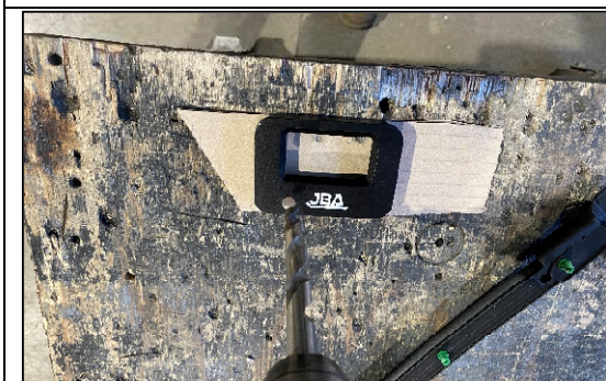
STEP 1.2.3 TURN THE FASCIA OVER AND COMPLETE DRILLING HOLE ALL THE WAY THROUGH. TAKE YOUR TIME, DRILL SLOWLY AND STOP FREQUENTLY TO ENSURE PART DOESN'T SPIN WHILE DRILLING.
